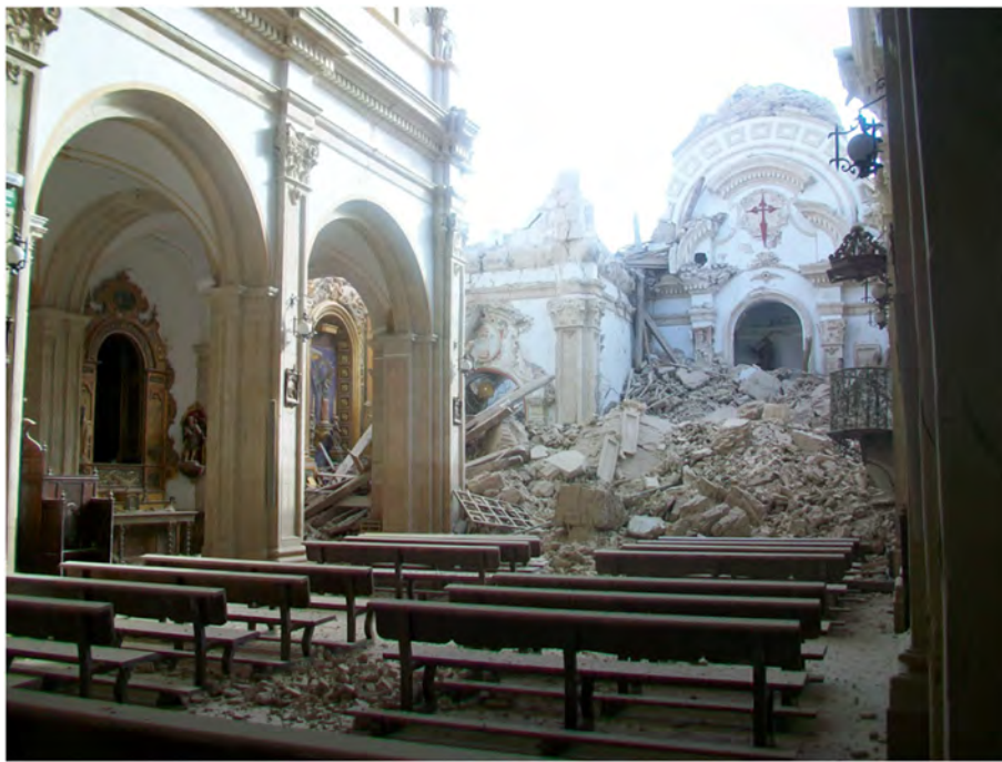
Fig. 14. Destruction in the church of Santiago resulting from the 2011 M_w 5.1 Lorca, Spain, earthquake ( https://en.wikipedia.org/wiki/2011_Lorca_earthquake ).
